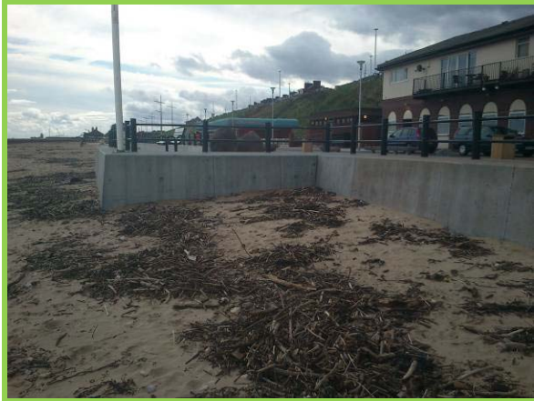
Low concrete encased wall at Marine Walk in good overall condition (Asset ref. No. 121AB901B0605C02)
