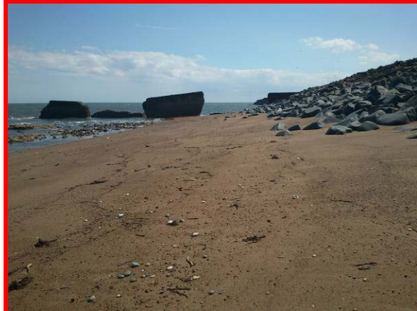
Remains of derelict concrete groyne from north (Asset ref. No. 121AB901B0801C01)
