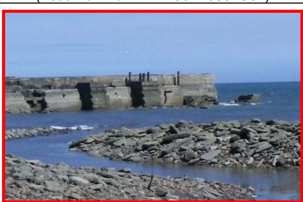
North East Pier roundhead has lost further material since 2010, photo 16.05.2013 (Asset ref. No. 121AB901B0801C04)
