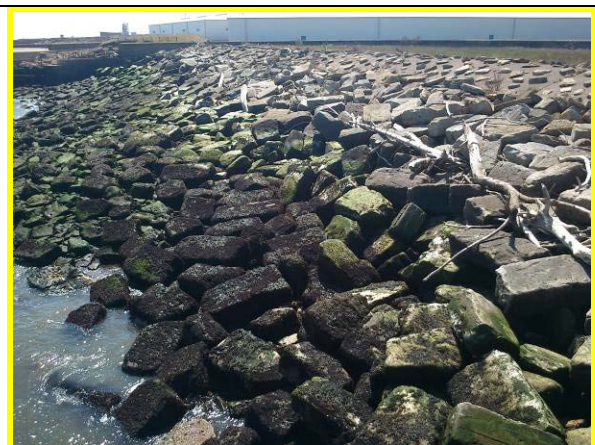
View of revetment from north, showing grouted concrete crest and secondary wall set back to rear. (Asset ref. No. 121AB901B0703C03)
