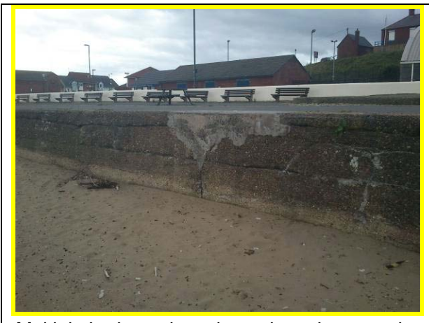
Multiple horizontal cracks and previous repairs in concrete wall (Asset ref. No. 121AB901B0702C01)
