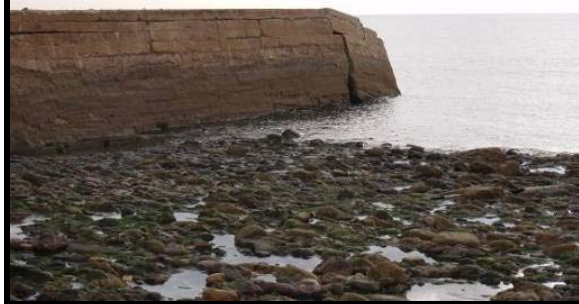
Failed seaward end of breakwater at south of port area. Photo from 2010 report. (Asset ref. No. 121AB901B0803C02)
