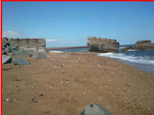
Remains of derelict concrete groyne from south (Asset ref. No. 121AB901B0801C01)
