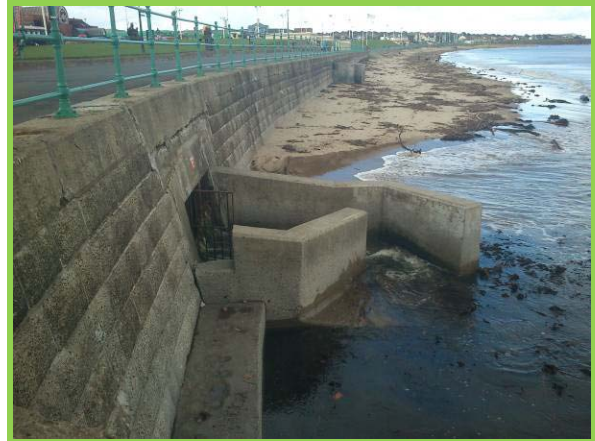
Outfall structures with cracks adjacent to wall. (Asset ref. No. 121AB901B0603C02)
