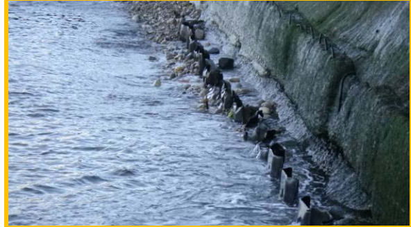
Highly abraded and corroded toe piling (Asset ref. No. 121AB901B0803C02)
