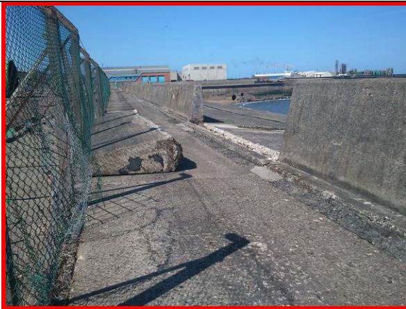
Failed section of crest wall. (Asset ref. No. 121AB901B0802C01)
