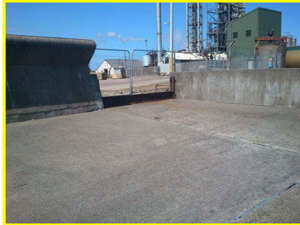
Gap in crest wall with missing flood boards (Asset ref. No. 121AB901B0802C04)
