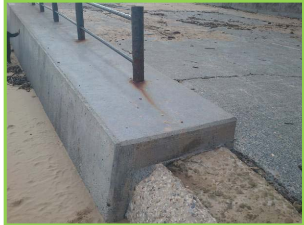
Corroded handrails adjacent to ramp at north which has cracks as reported in 2010. (Asset ref. No. 121AB901B0605C02)
