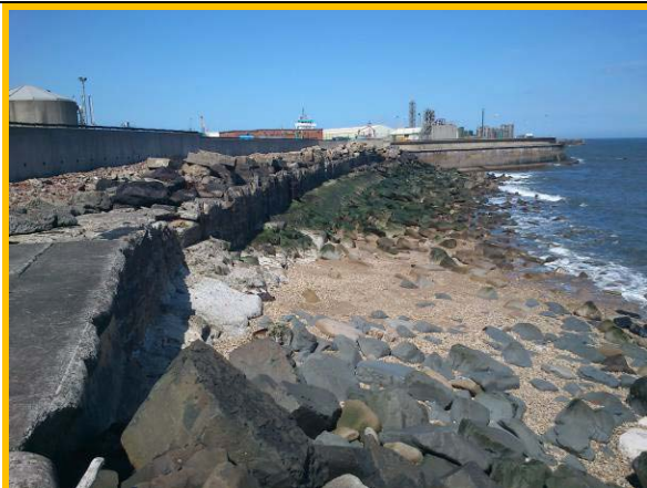
Loosely stacked rock armour on crest and at toe provides limited protection (Asset ref. No. 121AB901B0802C03)
