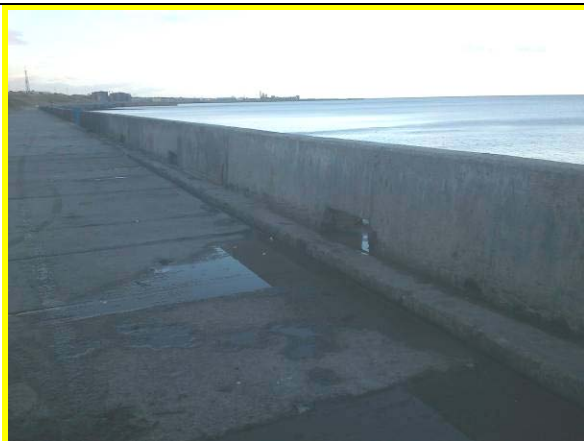
Crest wall with enlarged drainage holes towards southern end of defence. (Asset ref. No. 121AB901B0803C02)
