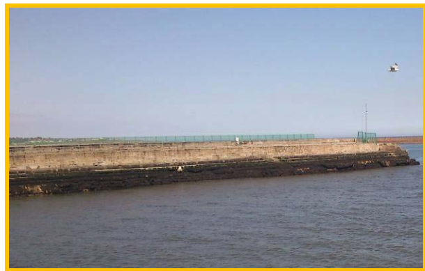
Voids in apron and undercutting of Old North Pier (Asset ref. No. 121AB901B0702C03)
