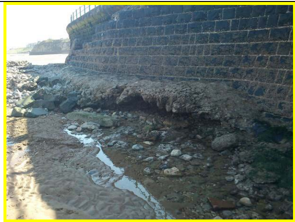
Undercut toe apron at disused set of steps (Asset ref. No. 121AB901B0604C02)
