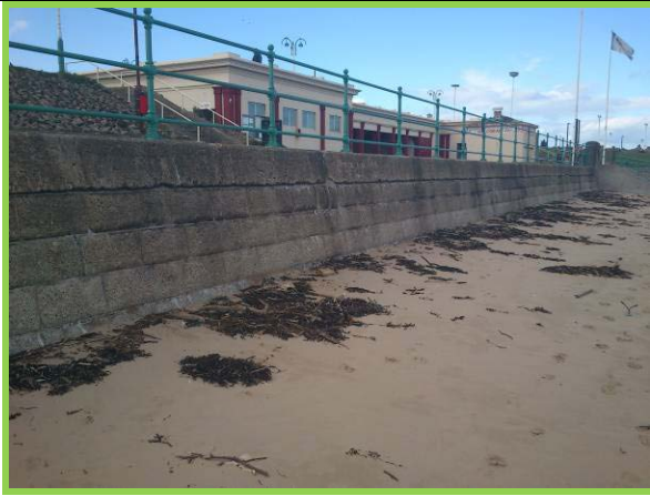
North end of seawall adjacent to Dykelands Road (Asset ref. No. 121AB901B0603C02)
