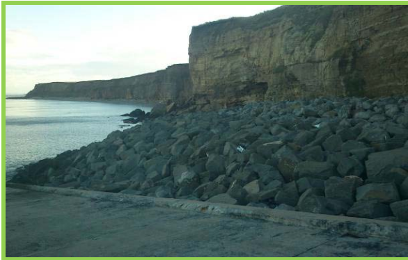
Rock armour at south end of Hendon Seawall with inactive cliffs in background. (Asset ref. No. 121AB901B0803C01)
