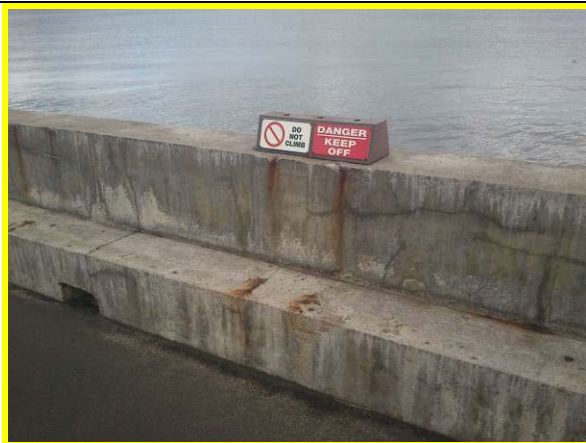
Crest wall with rust staining at fixings from previous seats and cracks (Asset ref. No. 121AB901B0603C03)
