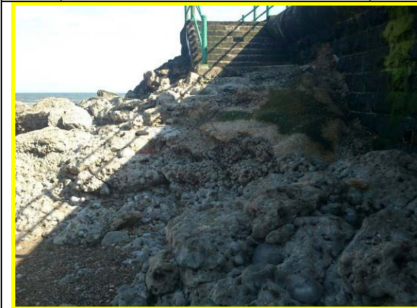
Eroded natural / grouted rock at access steps to Parsons Rocks (Asset ref. No. 121AB901B0604C02)
