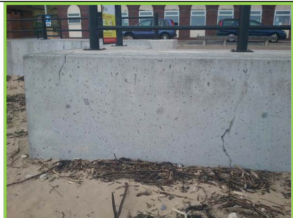
Minor vertical cracking in low concrete wall. (Asset ref. No. 121AB901B0605C02)
