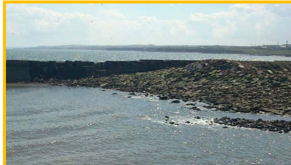
Random demolition rubble tipped into old dock to rear of South West breakwater (Asset ref. No. 121AB901B0802C06)
