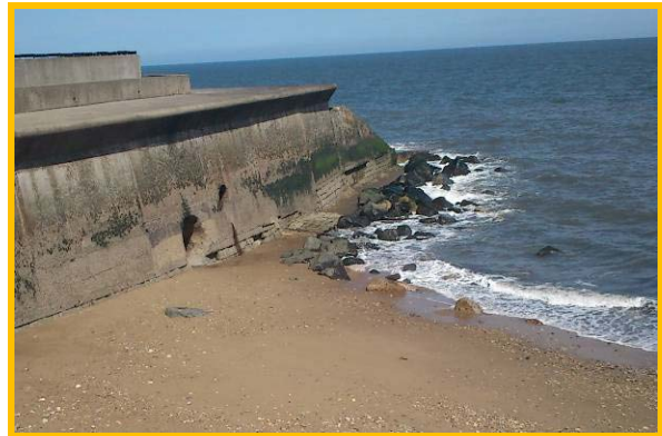
Damaged masonry and sheet piles require attention. (Asset ref. No. 121AB901B0802C01)
