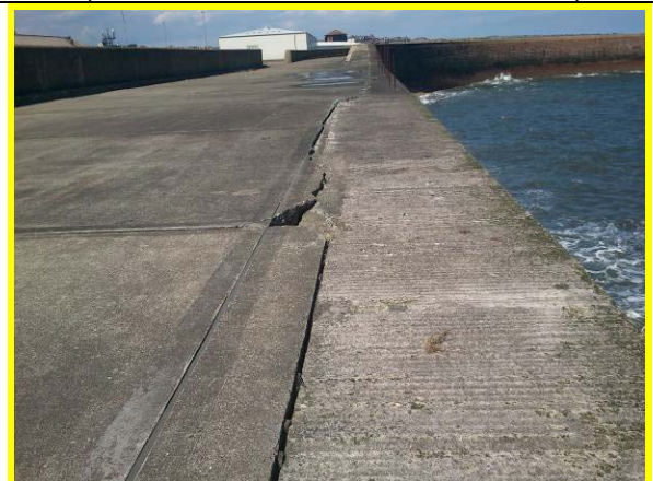
Slight lifting of deck slab (Asset ref. No. 121AB901B0801C03)
