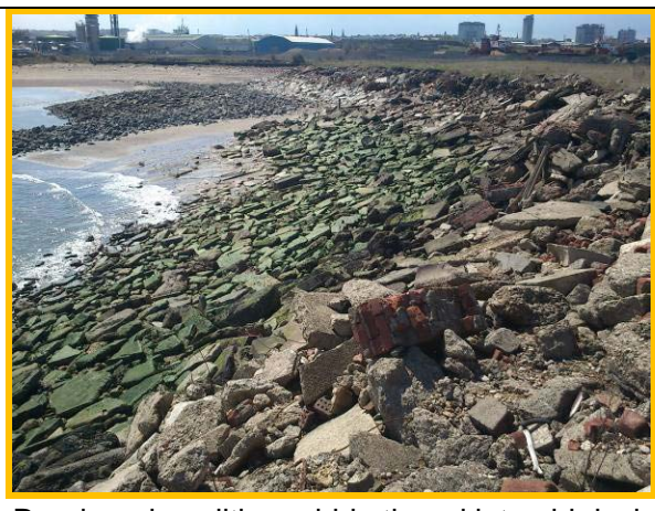
Random demolition rubble tipped into old dock to fill in front of buried quay (Asset ref. No. 121AB901B0801C08)
