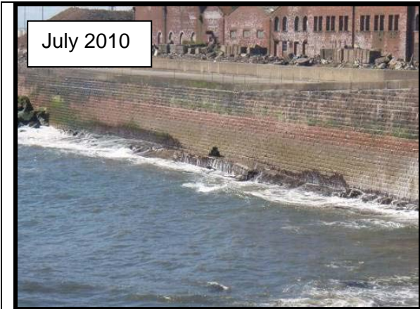
Void in base of wall – Photo from 2010 report (Asset ref. No. 121AB901B0801C03)
