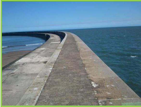
New South Pier in good overall condition. Deck slabs repaired since 2010 (Asset ref. No. 121AB901B0703C01)
