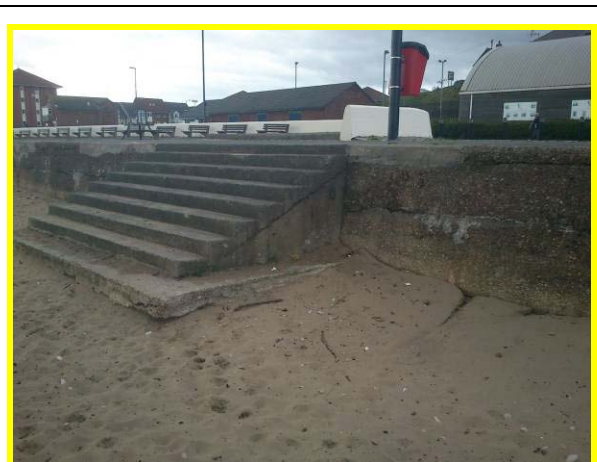
Undercutting at steps to Roker beach (Asset ref. No. 121AB901B0702C01)
