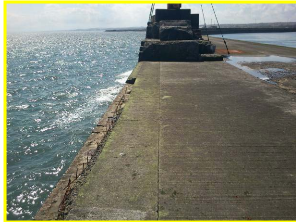
Missing section of coping near seaward end (Asset ref. No. 121AB901B0703C01)
