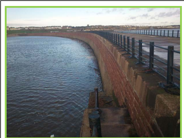
Inside face of Roker Pier appears in good condition (Asset ref. No. 121AB901B0702C04)
