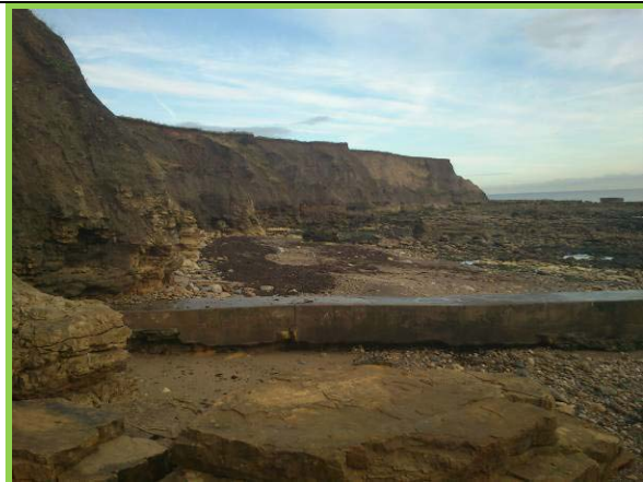
Mud slides in upper till cliff. (Asset ref. No. 121AB901B0804C03) Also shows undermined concrete cladding on outfall structure at Ryhope Nook.
