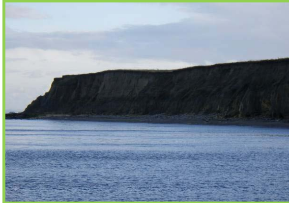
Cliffs south of Hendon are afforded a degree of natural protection by rubble at toe (Asset ref. No. 121AB901B0803C01)
