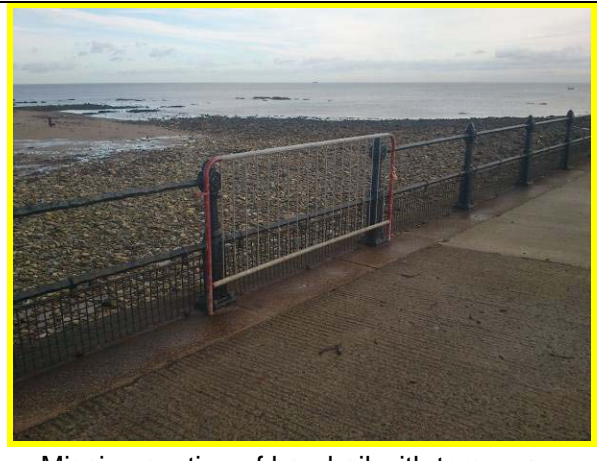
Missing section of handrail with temporary fence in place on north side of Roker Pier (Asset ref. No. 121AB901B0702C04)
