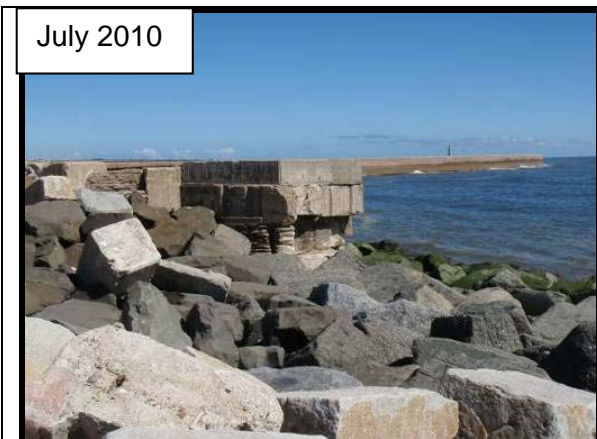
South end of wall protected by rock armour – photo from July 2010 (Asset ref. No. 121AB901B0801C03)
