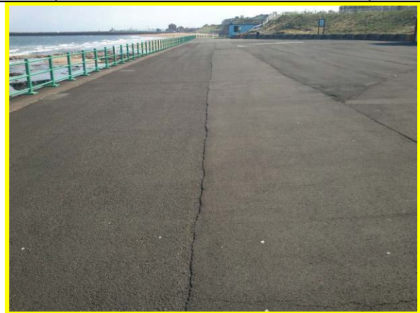
Promenade surface joints need resealing at Parsons Rocks (Asset ref. No. 121AB901B0604C02)
