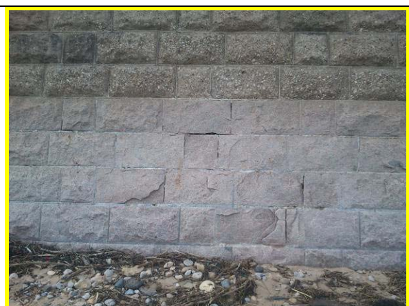
Localised abrasion / impact damage at toe of high masonry wall (Asset ref. No. 121AB901B0605C01)
