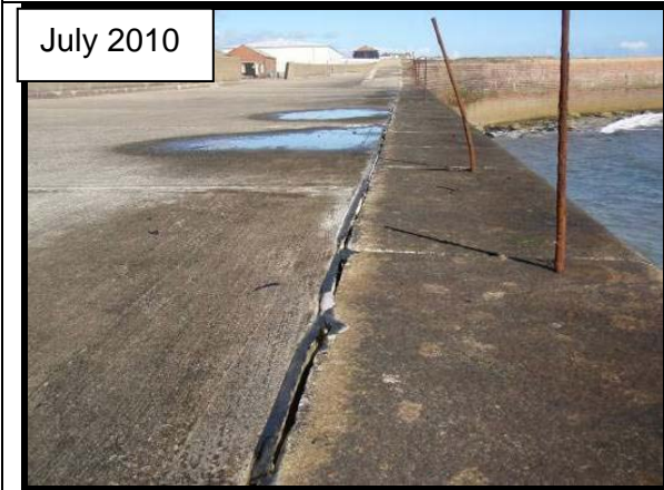
Deck slab above void – Photo from 2010 report (Asset ref. No. 121AB901B0801C03)
