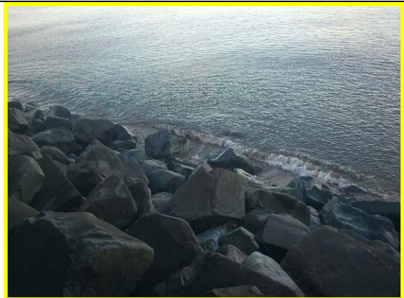
Localised displacement of rock armour at toe.
