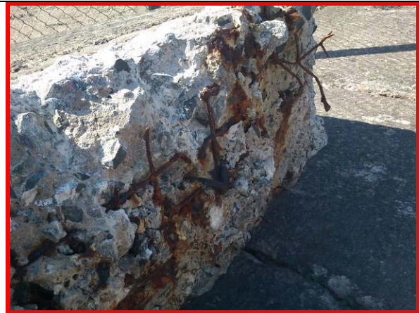
Close up of base of failed section of crest wall. attention. (Asset ref. No. 121AB901B0802C01)
