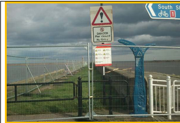
Old North Pier closed to public due to unsafe condition. (Asset ref. No. 121AB901B0702C03)
