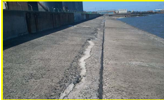
Cracking to crest slab with previous repairs and previously replaced sections of rear wall. (Asset ref. No. 121AB901B0802C01)
