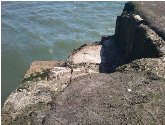
Missing section at head of New South Pier (Asset ref. No. 121AB901B0703C01)
